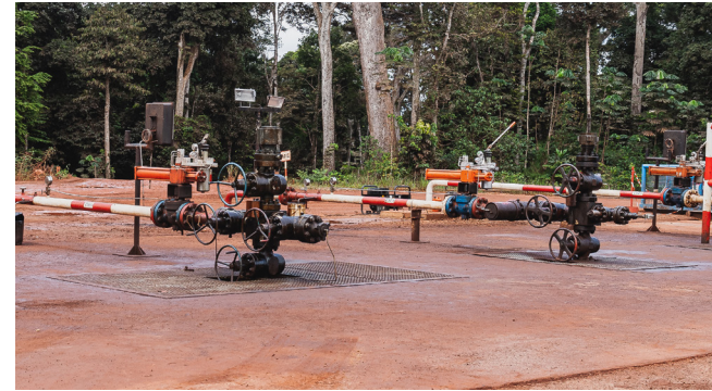
AUTOMATED GAS VALVES
