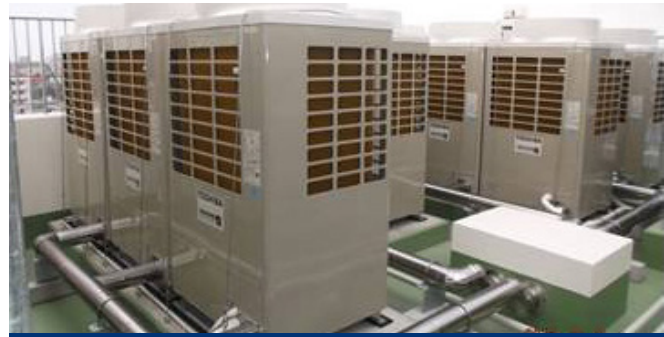
HVAC SYSTEM PRESSURE FOR SUPERHEAT MEASUREMENT
